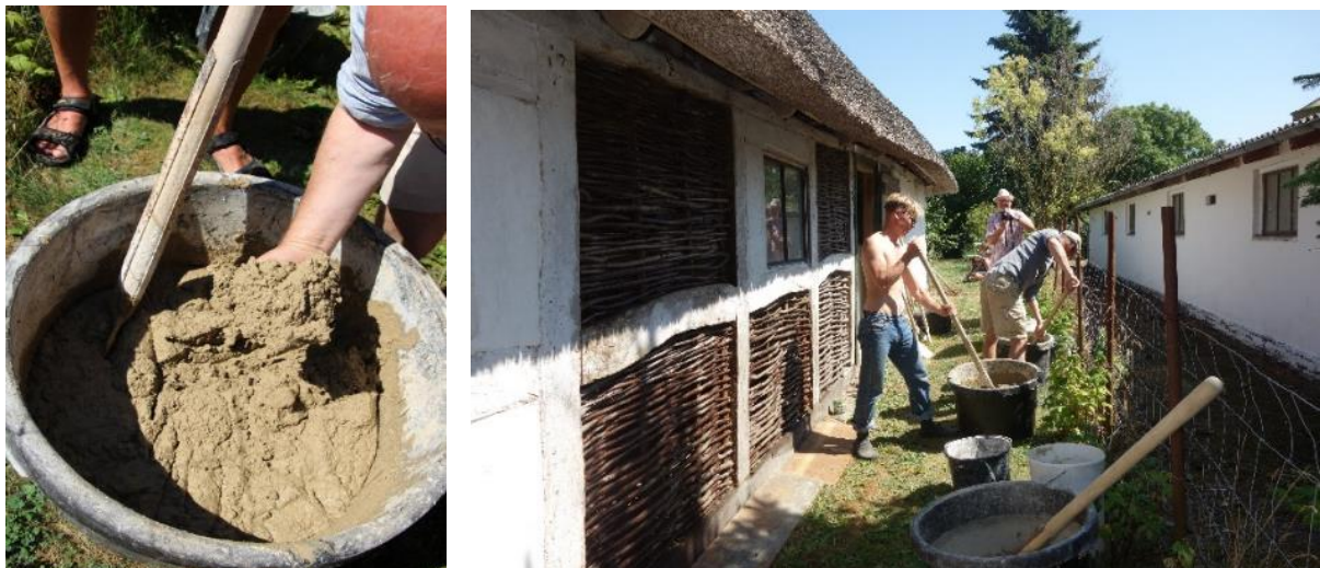
Figure 7. A tub of ready mixed clay mortar, ready for use as wattle and daub. Photo: Søren Vadstrup.
