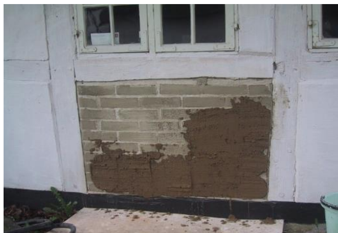
Figure 5. Repair of a fallen plaster on the adobe klay wall. Photo: Søren Vadstrup.
