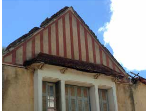
FIGURE 5 The ruins of Chacara das Rosas in the city of Cambuquira, about 2014.
