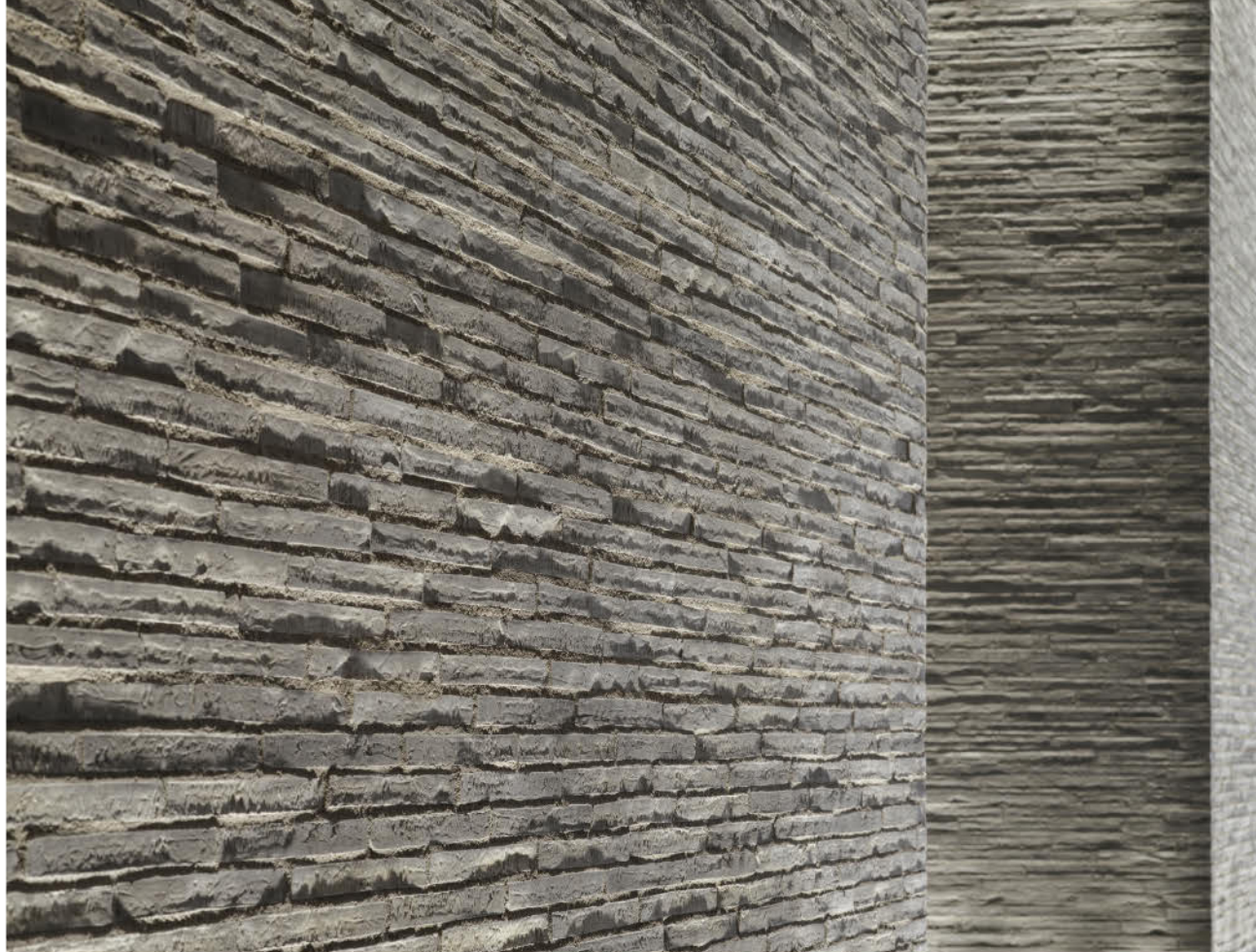
“Wall grazing” highlights the irregularities of the handmade bricks and dramatises the texture of the lobby walls.
