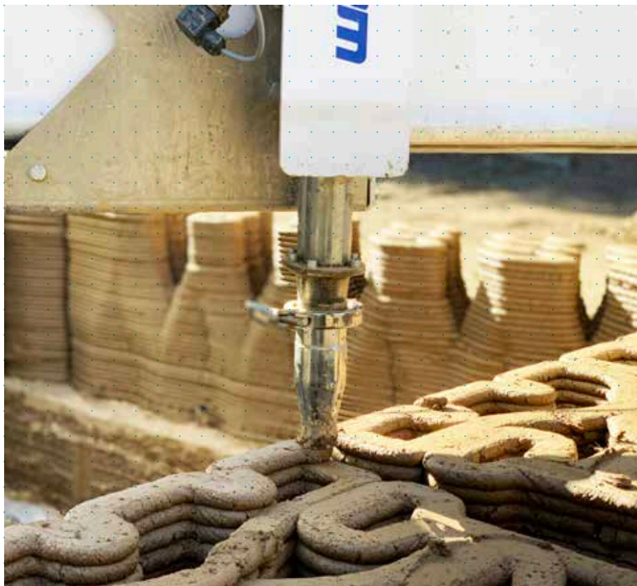
30cm per day of wet earth are extruded onto the printed wall. Drying takes several days and determines the rhythm of the printing process.
