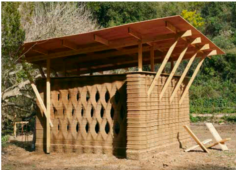
TOVA, the first earthen 3D-printed building in Spain, was printed by the students of the 3DPA programme over six weeks in February 2022.
