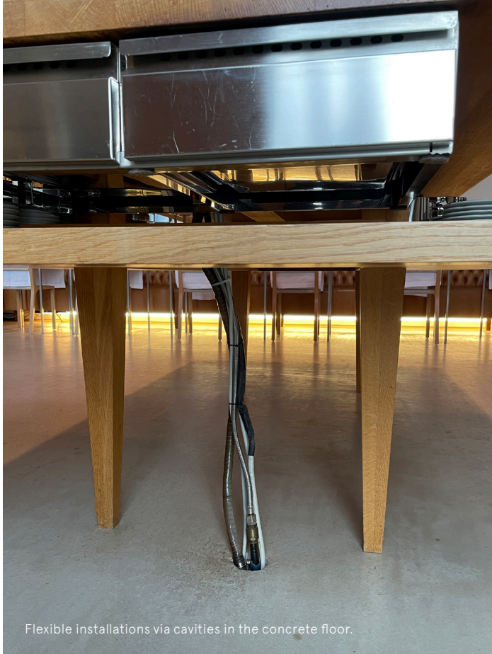
The utilities can be reached by removing a wooden plank along the interior wall of each office.
