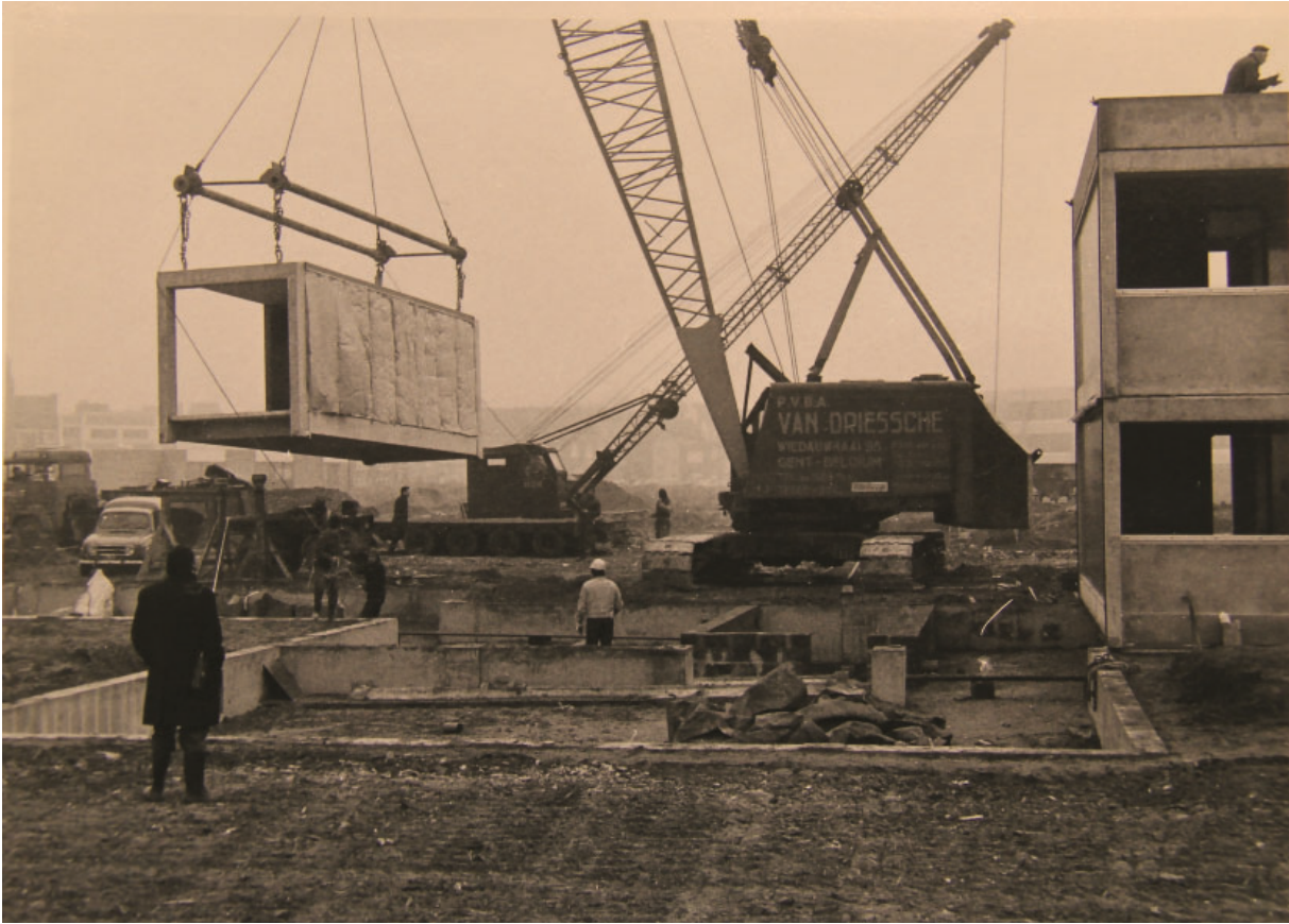
Fig.1, Delivery of the modular units for the construction of the student homes at the VUB campus in Elsene in 1973 – © Archive of the Technical Service 'Infra' of the Vrije Universiteit Brussel.
