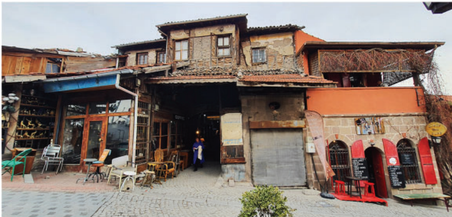
Fig.2: The Main Entrance on the West Façade of Pilavoğlu Han Photo by the Project Team, E.M.Kısaer Koca
