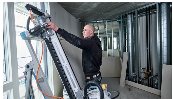
Fig 2.14 The Kobot system being used on the construction site to cut drywall panels, 2022 © Kobots.
