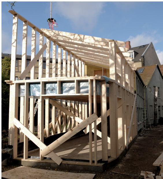
Fig 3.4 The Olaf Ryes Gade project after the structure was erected in one day in 2020, Odense, Denmark.
