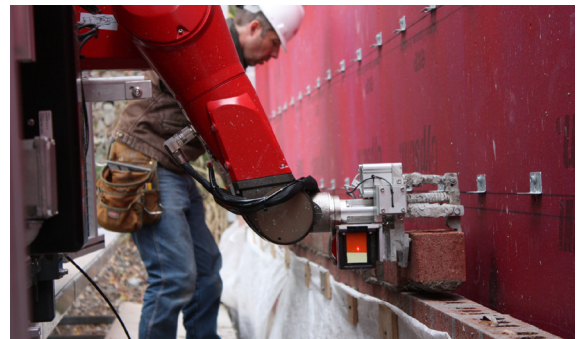
Fig 2.13 The brick-laying robot SAM on the construction site working in conjunction with brick layers, 2017, © Scott Peters, the image of the SAM system.
