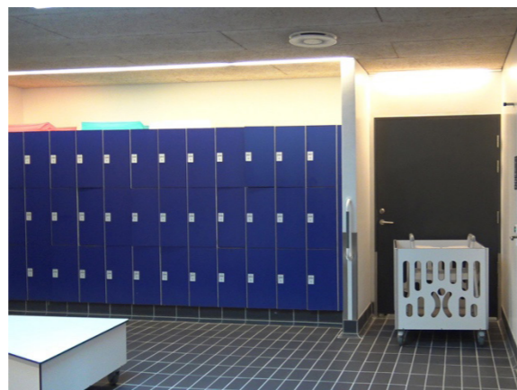
Figure 6.1-25 Vandhalla: linear lighting elements over the lockers and the door
