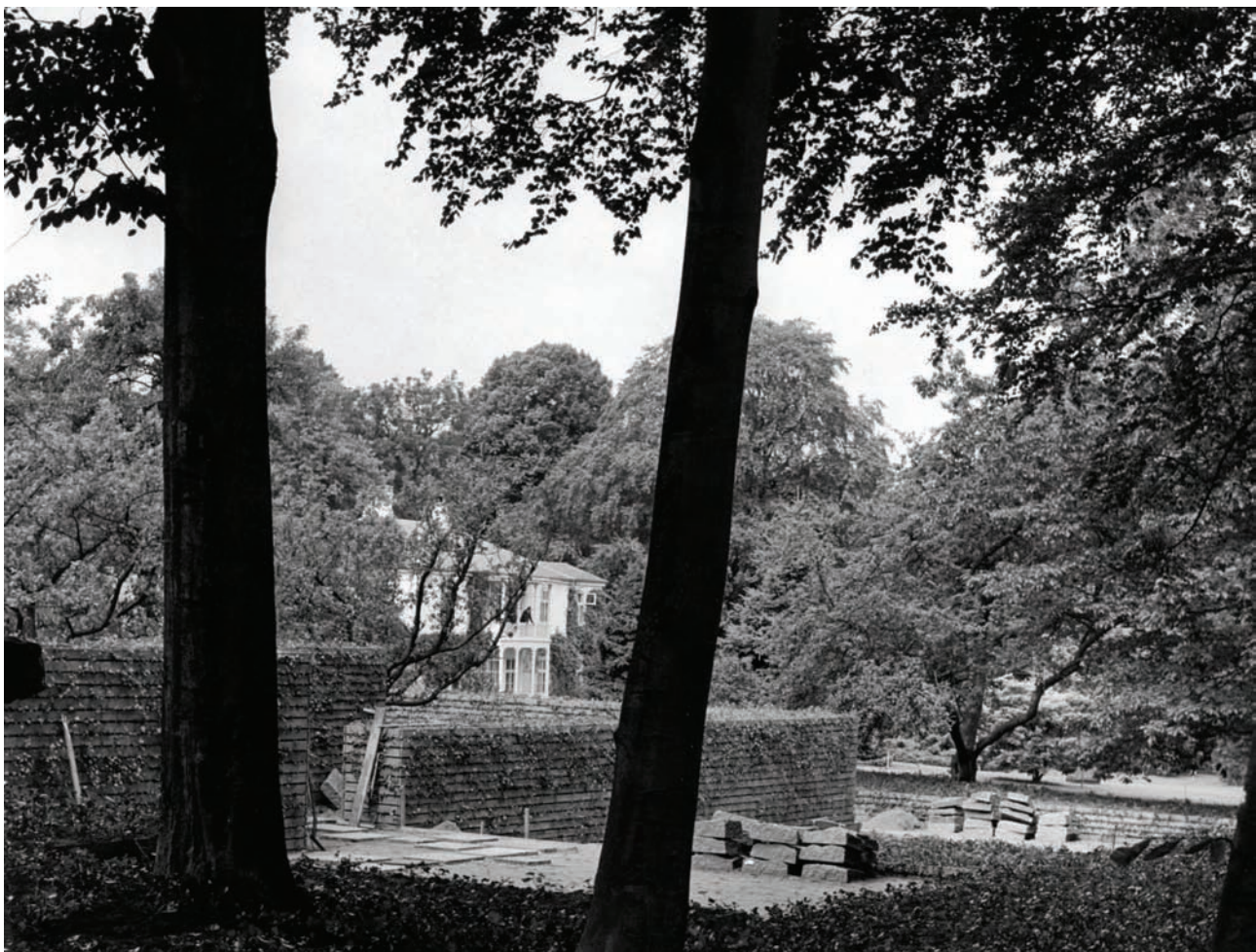
3.22 View of the sculpture terraces under construction, summer 1964, with villa in the background.
