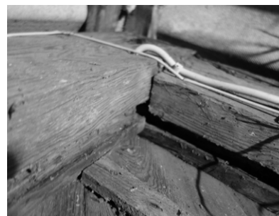
Figure 9: Construction detail at north-western gable. Here, the rafter is made from pinewood and provided with a groove originally intended for the attachment of gable boards. The pinewood rafter is typical to roof constructions and in contrast to the other rafters, presumably made from poplar. Photo, Thomas Kampmann, 2019.
