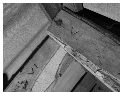
Figure 10: The top joint of rafters in the roof construction in the apprentice house. The timber mark, here on rafter no. VI, indicates a seven-bay house of two gable in pinewood rafters and 6 numbered rafters in between in poplar. Photo, Thomas Kampmann, 2019.
