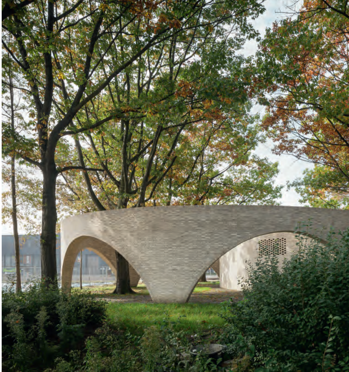
The three electricity substations that power the Brabo 2 tramline in Antwerp feature brickwork of exceptionally high quality.
