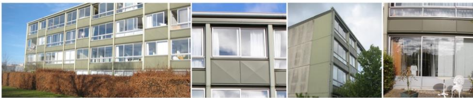
Figure 8: The south facades have large balconies. At the time of the investigation the facades were being demolished due to renovation works. The facades have clear potentials for reuse in new building layouts. Illustration Martín Jiménez.
