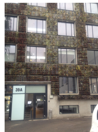
Figure 4.34 Failed green wall: Example of an unsuccessful green wall in Aarhus, Denmark, removed in 2015
