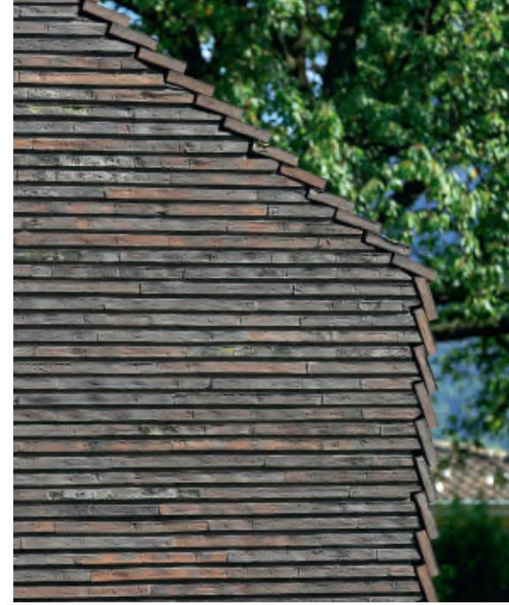
The Kolumba gables have been carefully cut in such a way as to interlock with the bricks on the roof and façade. The result is both minimal and highly detailed.
