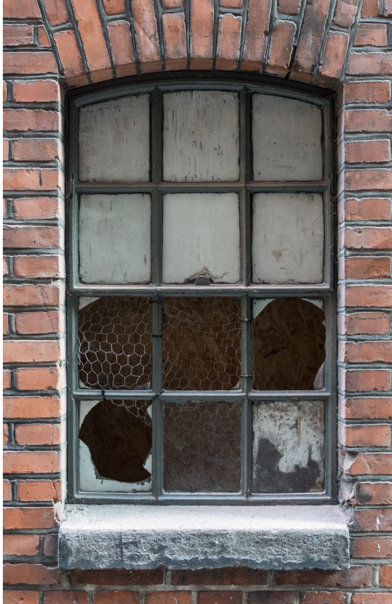
A devastated window in the alley. Multiple materials and textures and the passage of time create a complex scenario.
