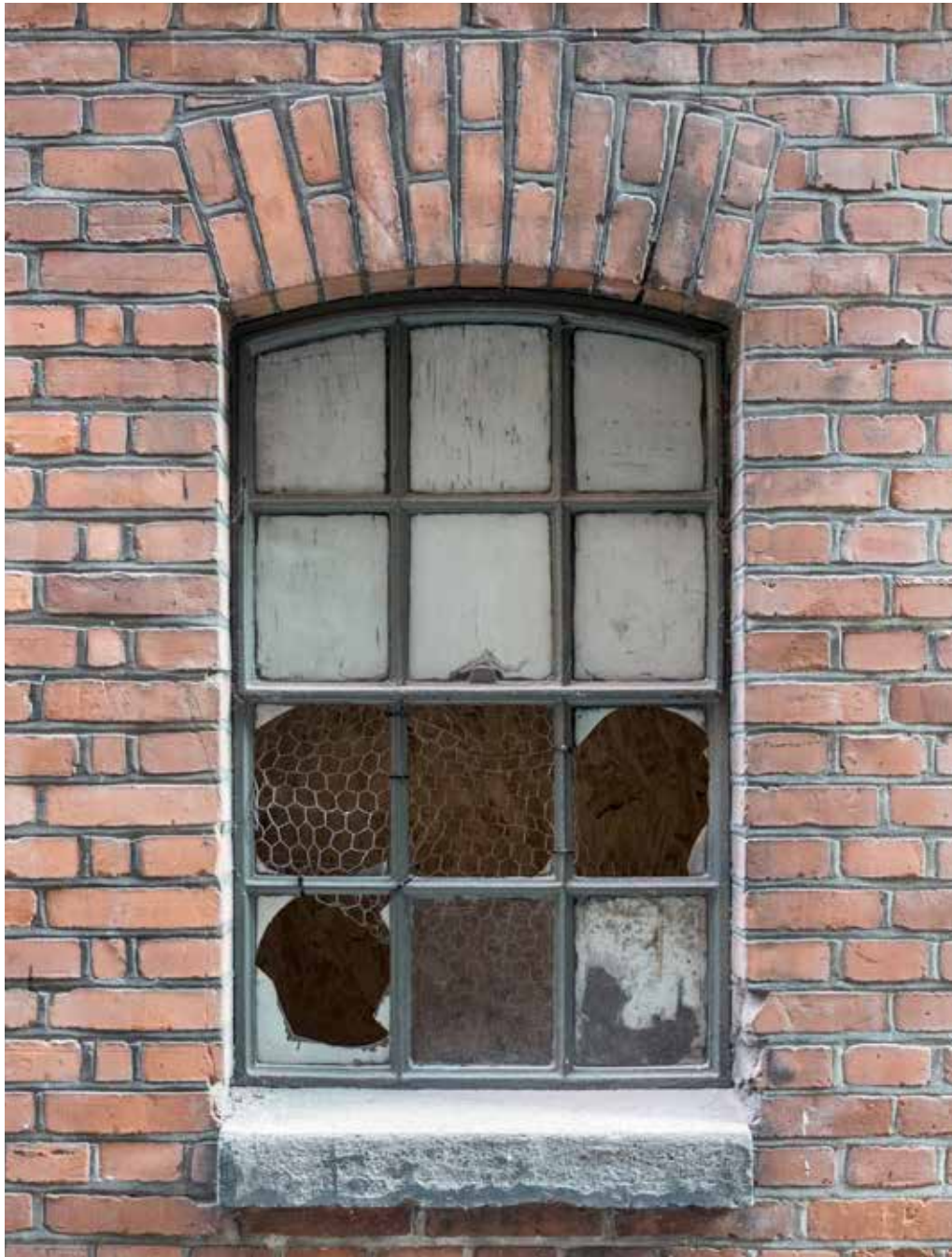
A devastated window in the alley. Multiple materials and textures and the passage of time create a complex scenario.
