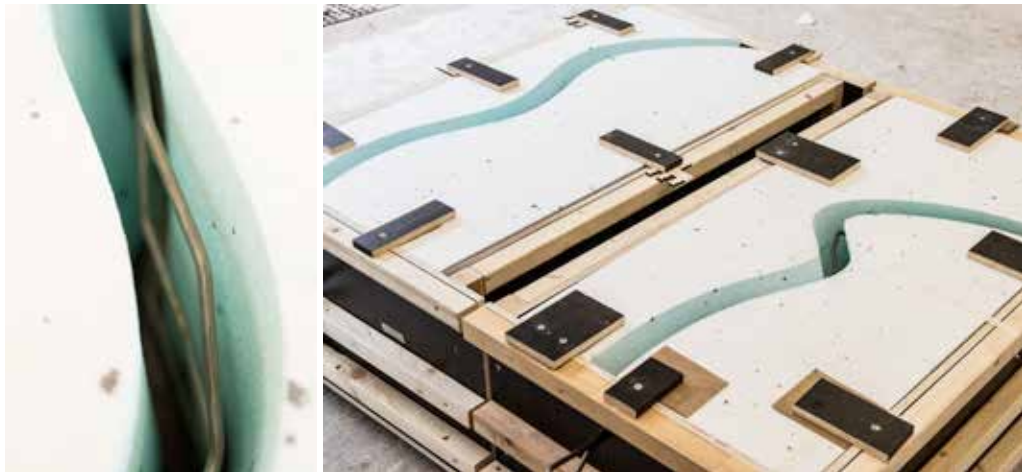
Formwork with rebar fixed inside, ready for casting. The formwork surface is treated with retarder to make demoulding easy despite of the curvy shapes.
