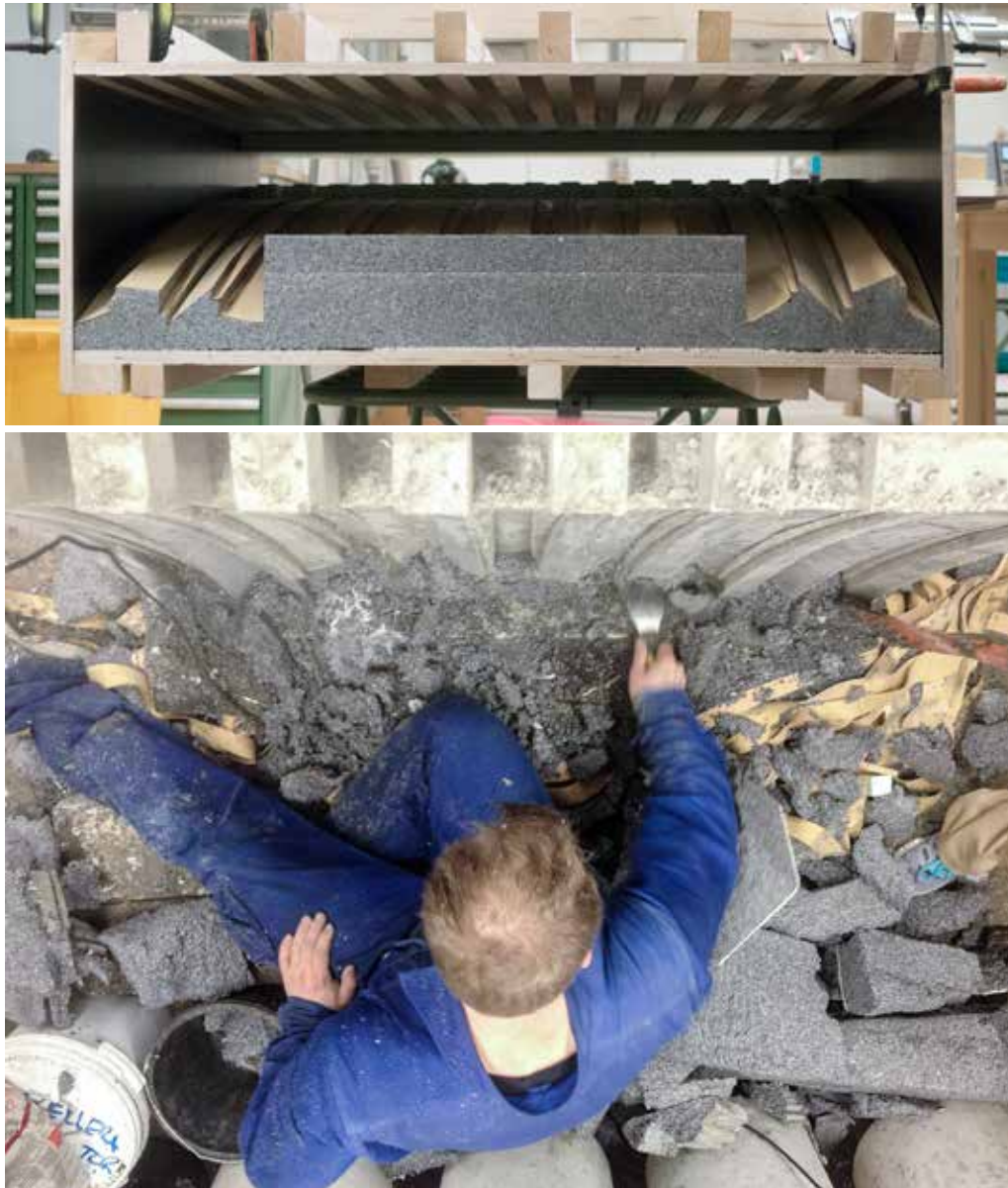
Upper: Formwork almost ready for casting. Different surface treatments are applied. Lower: Formwork removal reveals the different surface textures.
