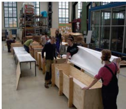
Assembling the formwork. Mounting the inside polystyrene moulds in an outside load bearing structure of plywood and rafters.
