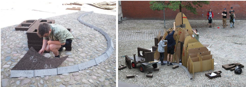
Figure 4: Construction of the vault (Left) Test-fitting the voussoirs. (Right) Constructing the cardboard centering.
