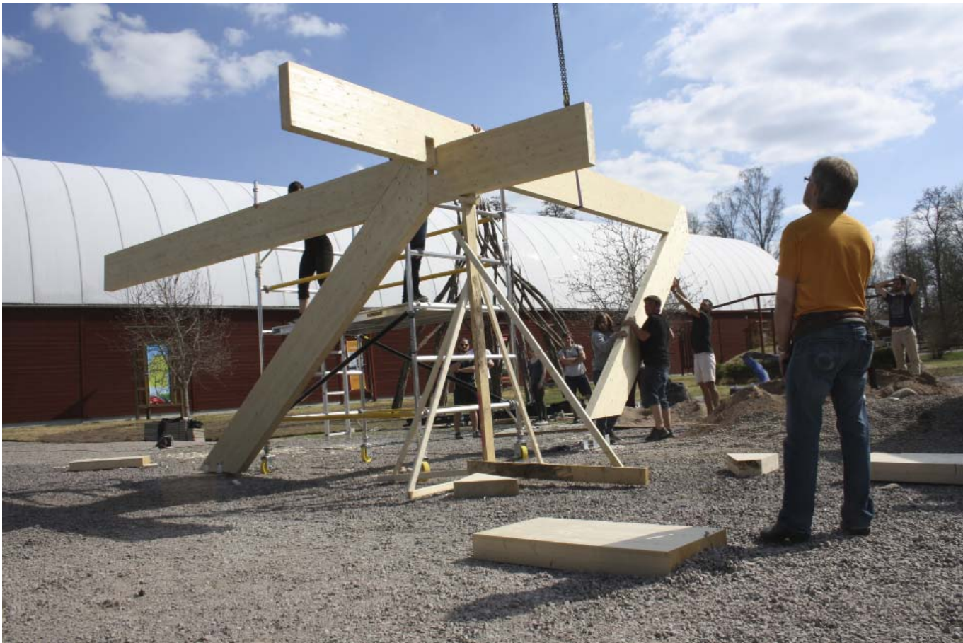
Jacob Stålgren from Bygg & Handel would help us hoisting the elements together for the 'Span and Mass' project.
