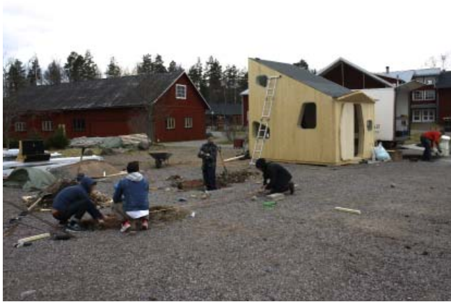
5 days before the workshop began, Nikolaj Callisen Friis went to Virserum with four students from the 'Span and Mass' group to cast two 200 litre foundations (using around 900 kg of concrete). This had to be done in advance in order for the concrete to cure.
