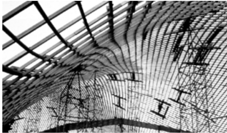
Figure 9: The process of erecting the structure was a complex task of gradually raising the supporting scaffolds and moving the lifting points, depending on the behaviour of the mesh.
