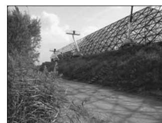
Fig 5C: Acoustic Barrier, ONL [Oosterhuis_Lénárd] 2004, Building site progress, 15 September 2004, the Cockpit will connect to the left end
